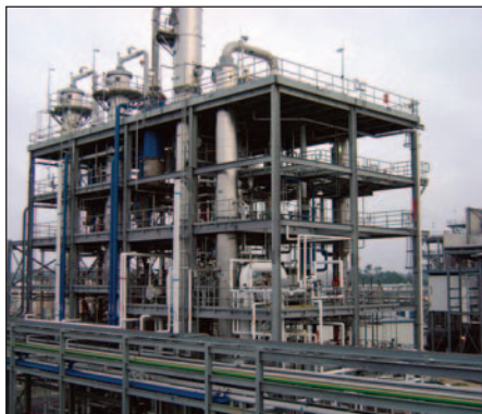
Field installed equipment and piping. A turnkey project.
