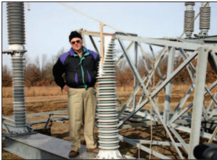
GRDA Substation Engineer Bud Averill surveys the damage inside GRDA's Highway 412 Substation following the January '07 ice storm. Most of GRDA's damage in January '07, was well east and south of the MidAmerica Industrial Park.
