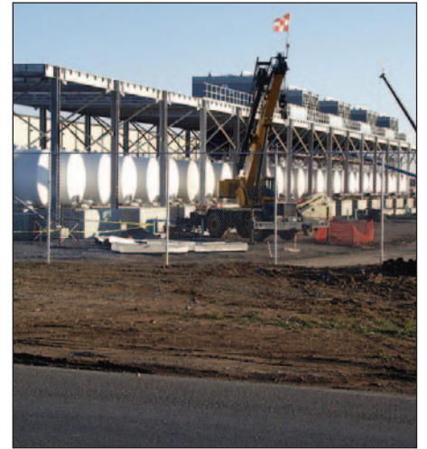
Construction proceeds at the Google facility just across from the new Gatorade plant.
