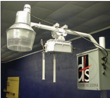
One of the Cisco Access Points (AP) used to generate a wireless signal. At right, a battery backup that can be used with the AP to generate up to 40 hours of power if there was a power outage.
