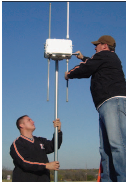
James Cavin (left) and Brian Ledbetter (right) install a rooftop mesh access point for the Pryor network. Access points like these are used to send out the wireless signals from the network that DTS is creating.
