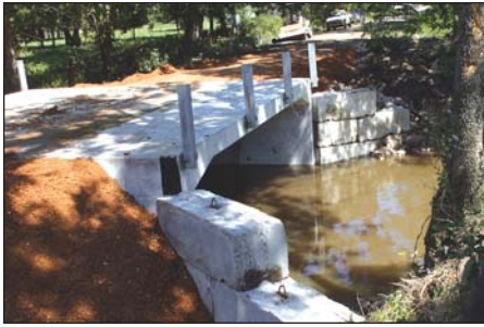
A new Wolf Creek Bridge was reconstructed as a result of the partnership between the Cherokee Nation and Mayes County Commissioner Alva Martin. The project is another example of how the Nation invests in sustainable community development such as better roads and bridges.
