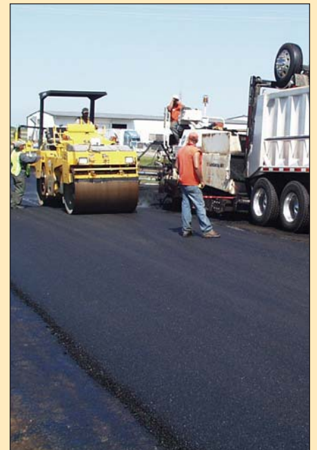
A crew from Horizon Construction of Owasso applies asphalt to the new Airport Road at MidAmerica. The now completed project replaced a curved road to the MidAmerica Airport with a new 32-foot wide straight version that created a new intersection with Webb Street. Other components of the project include shoulder widening, the creation of a new drainage system and raising the grade to each side of the GRDA rail spur.
