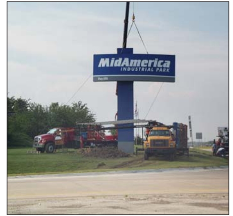
A crew from Claude Neon Federal uses a crane during the installation of one of the primary entrance signs.
