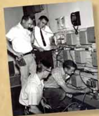
Presidential visits demand security and communications capability at all times. LBJ's visit to MidAmerica was no different. The Secret Service oversees last minute testing of phone room wiring.
