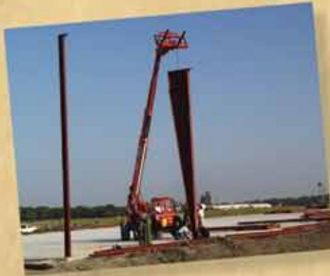
Red iron forms the support frames for the new Solae warehouse and distribution facility.
